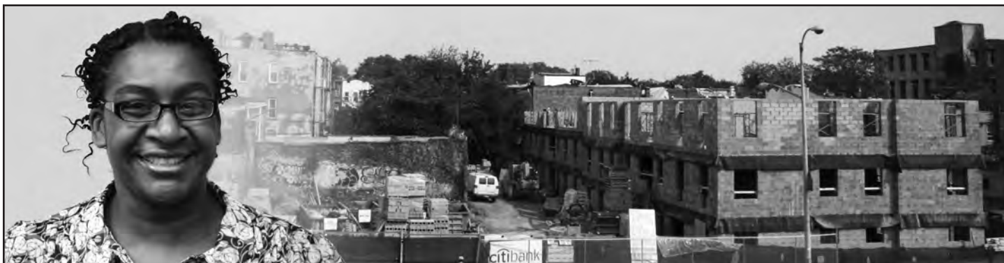
New family partners are joining volunteers who are hard at work on our Atlantic Avenue complex. Top left, Board Member Suzette Hunte saws metal pieces with the assistance of AmeriCorps member Andrea Nadel. Top right, site staff check architectural plans. At bottom is an expansive view of the Atlantic Avenue site, with new family partner Zericka Griffith in the foreground. Photos by Deborah Schwartz
